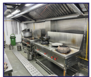
EXHAUST HOOD &/ DUCT
